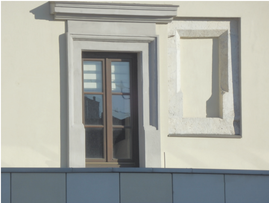
Fig. 17. The window frames that did not survive from that period were reconstructed. Frames from the same period in the Pauline Monastery in Priinczow were used as a model. Photo by M. Błażewicz
