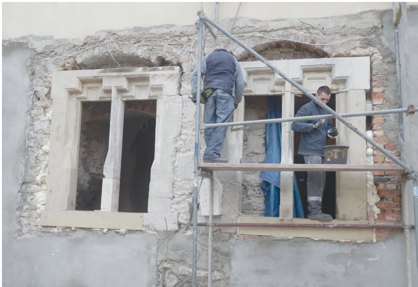
Fig. 12. Stone window frames in the eastern risalit — from the side of the cloister. Reconstructed on the basis of the preserved elements. The adaptation of historical details found during construction works could not be included in the project and thus did not fall under external funding. All such works had to be covered by the investor's own resources. Photo by M. Błażewicz
