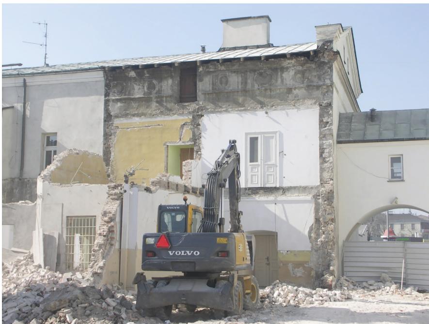
Fig. 9. Demolition of structures in poor condition that were added in the 19 th and 20 th centuries. The detail of the cornice in the historic monastery building was uncovered. Photo by M. Błażewicz
